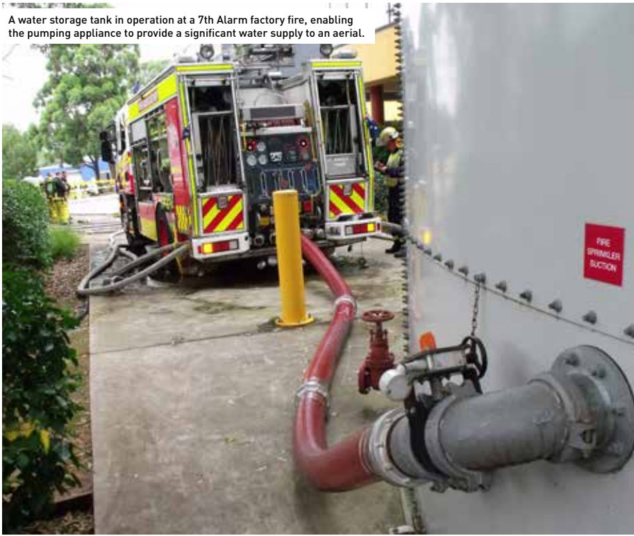
A typical water storage tank and brigade suction point, note no two are the same.
