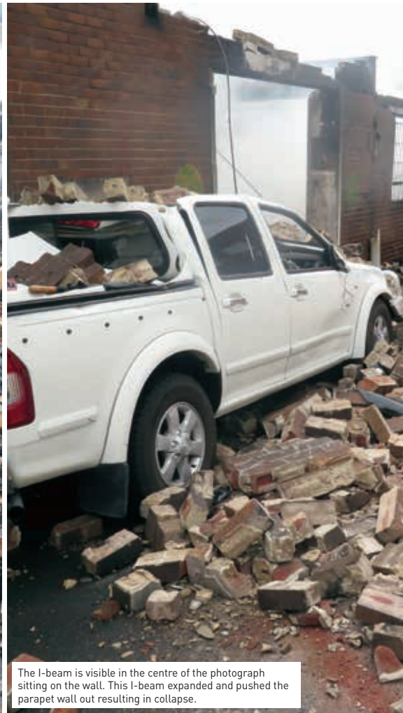
Aerial view of parapet wall collapse at Macquarie Street fire. The I-beam extending from front to rear of building had expanded due to exposure to flames, pushing the parapet wall out, causing collapse. Photo courtesy SO Wayne Schweickie FIRU.
