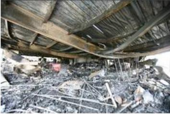
Figure 39 Structural collapse of building
